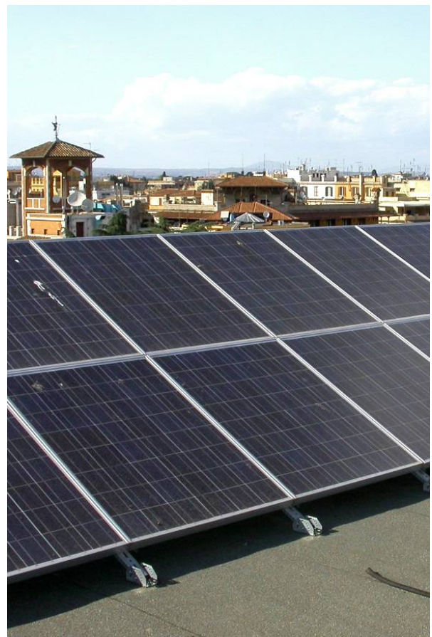
Photovoltaic solar panels (Image: Enel Green Power S.p.A.)
