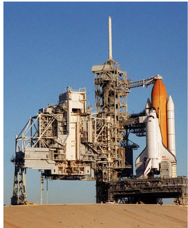
The Rotating Service Structure after rollback to the park position prior to launch of the STS-97 Shuttle Mission. (Image: NASA)
