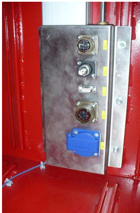
Figure 5.9 – Electrical connections inside gondolas
