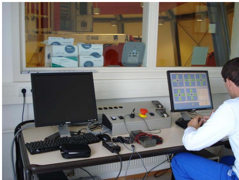
Figure 3.1 – Operation Control Station
