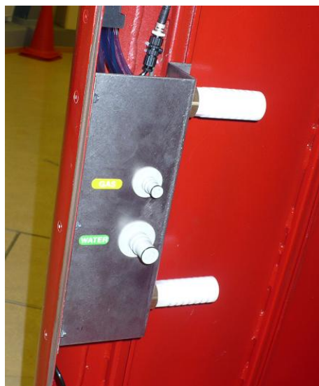
Figure 5.6 – Gondolas outlet sockets for Water and Gas
