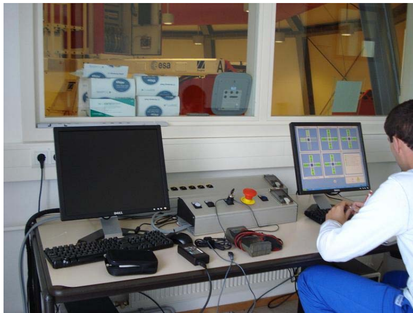
Figure 3.1 – Operation Control Station
