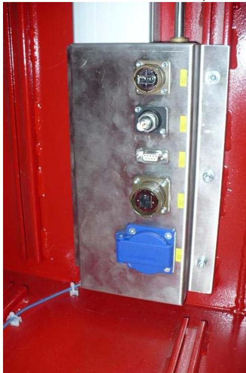
Figure 5.9 – Electrical connections inside gondolas
