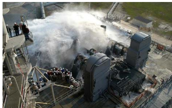
Sound Suppression System test on launch pad 39A at the Kennedy Space Center. (Image: NASA)
