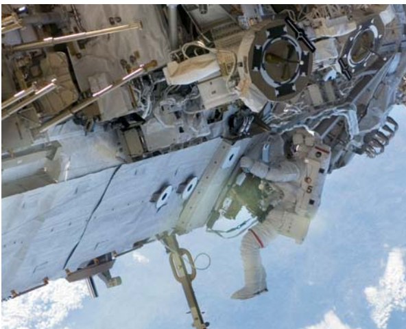
NASA astronaut Joseph Tanner connecting cables on 12 September 2006 during STS-115 mission, which installed the P3/4 truss onto the International Space Station. (Image: NASA)
