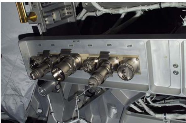
(Top) Connector panel on the S0 truss circled in red for reconfiguration of avionics. (Bottom) close up of left-hand side of connector panel. Power channels 2 and 3 configured through the two leftmost connectors shown during second EVA. Power channels 1 and 4 configured through the two rightmost connectors shown during third EVA. (Image: NASA)
