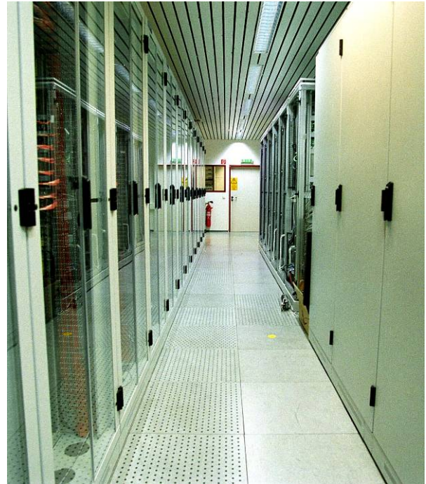
Network Equipment Room at the Columbus Control Centre. (Image: ESA)
